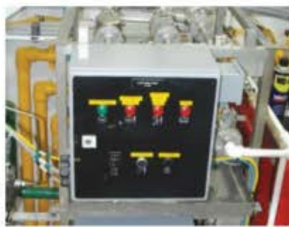
The Tier 4 selective catalytic reduction (SCR) emission control system requires its own space in the engine room.
