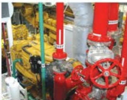
Two Caterpillar 3561E engines and emission control systems, plus pump engines and intakes for the firefighting system.
