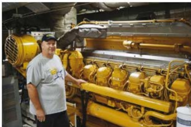
Capt. Jim engineer Michael Cobb stands alongside one of two Cat 3516E units delivering 3,386 hp each.
